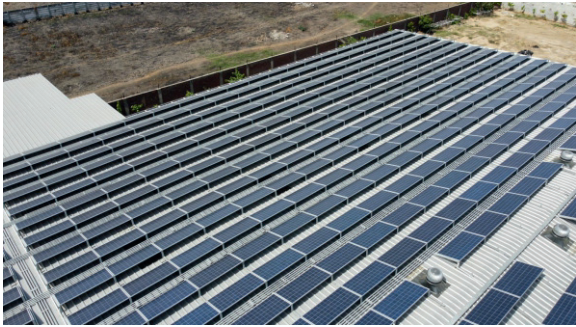
Solar mounting structure
